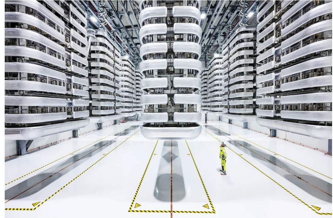
A Hitachi Energy HVDC VSC hall 5
