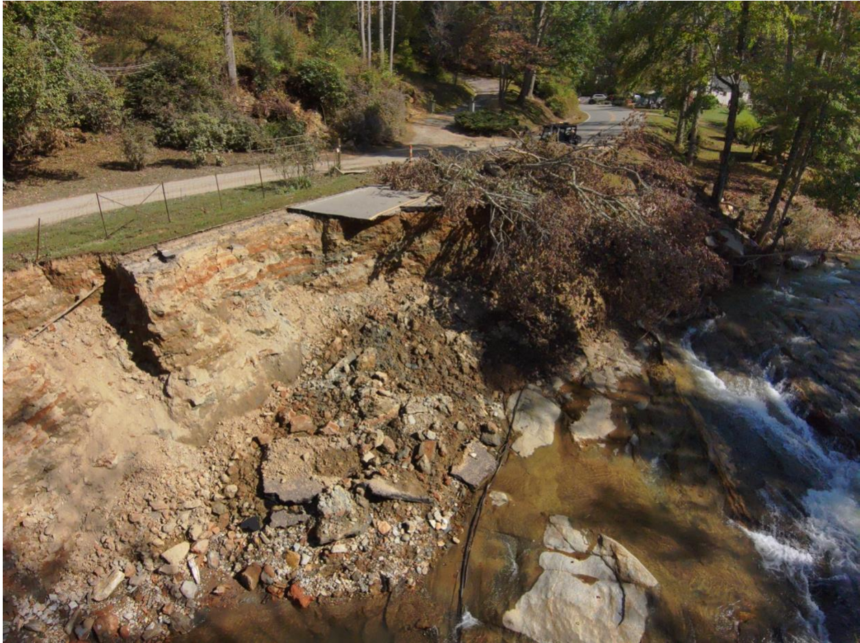
Figure 7: Bank and Road Erosion, NC Route 9, Buncombe County, NC October 8, 2024 (Credit: NCDOT)
