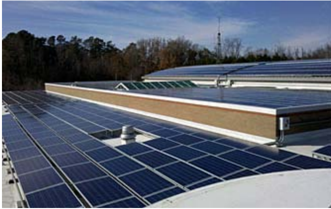
The solar power array at the N.C. Global TransPark
